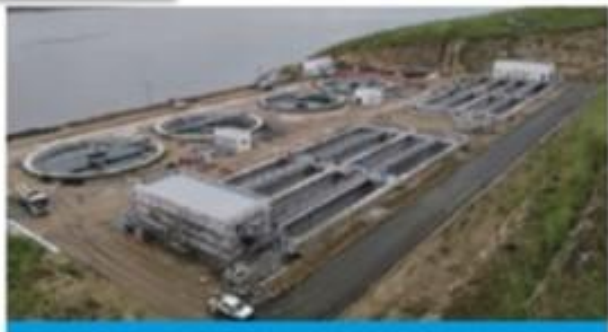
Papua New Guinea Sewerage PJ
